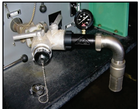
Figure 10. Pressure valve attached to the footvalve.
